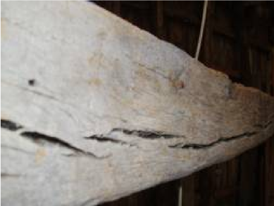
Large longitudinal checks on a wooden element (15 th -16 th century)
