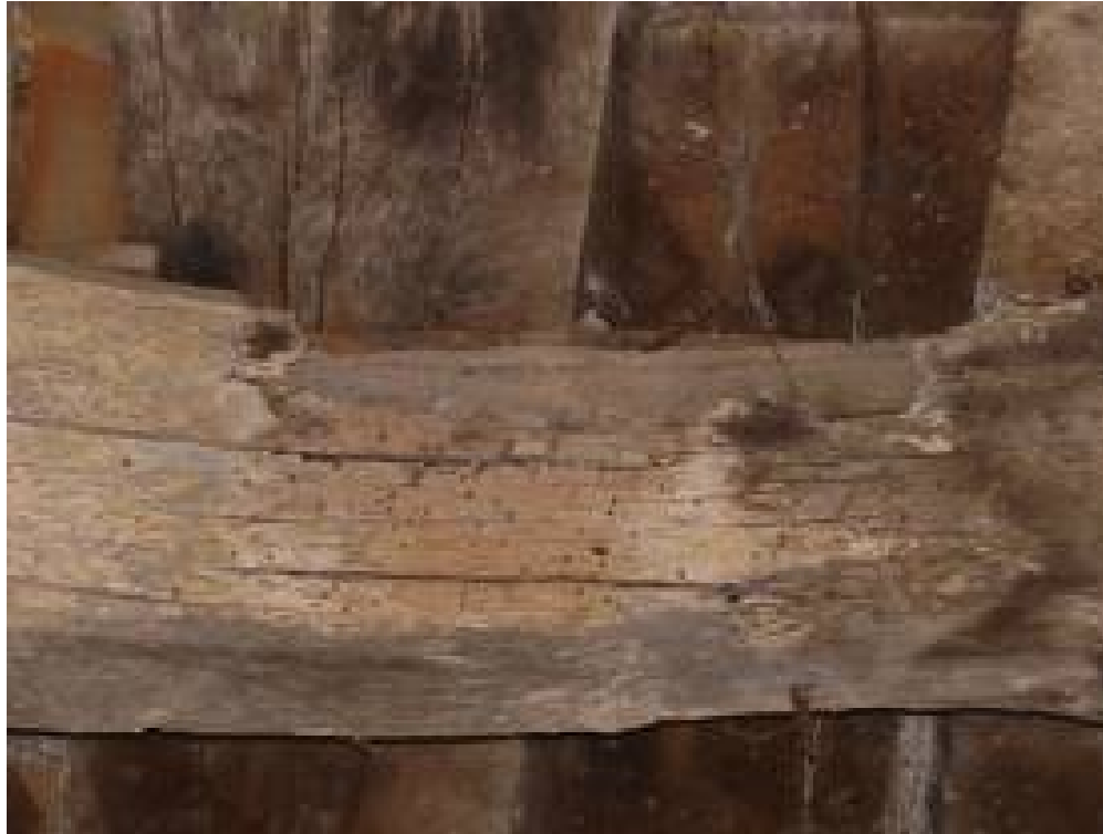
Rot and wormholes on the surface layer of an Oak structural element.
