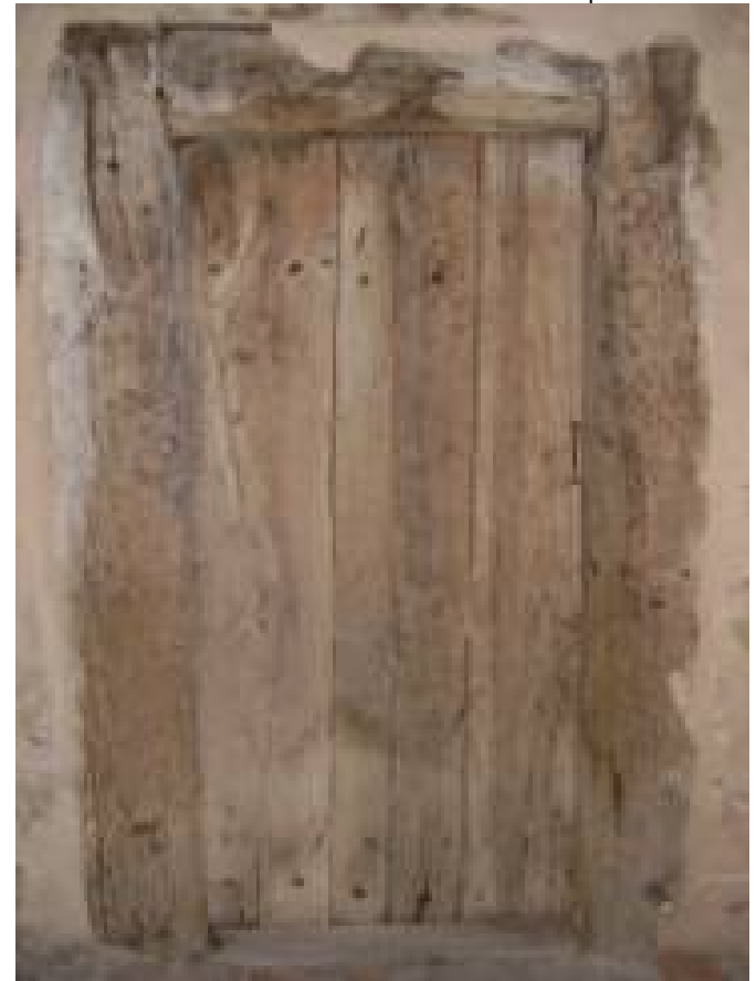
Oakwood door that needs conservation
